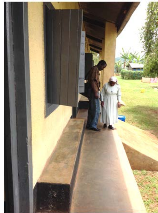
Renovations made in a PNFP facility in Kyenjojo district, using additional revenue from HBVP
