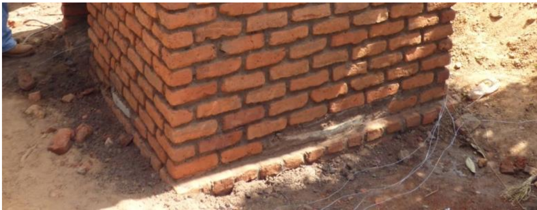
A latrine built with a foundation because the area chosen for the latrine was uneven and storm water could potentially affect the walls of the latrine.
