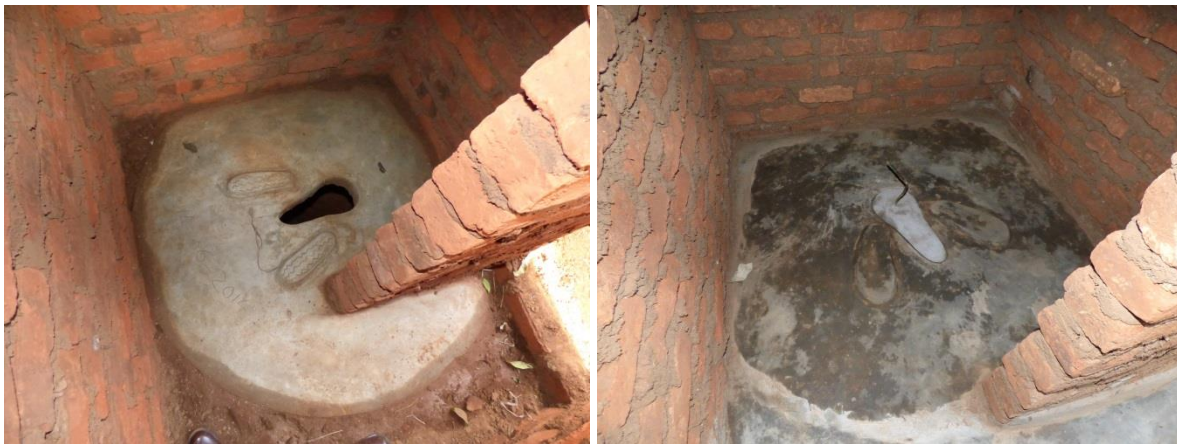
These photographs show a dome slab that is raised in the center (left) and a flat reinforced slab (right).
