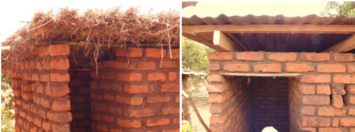
These photographs show a variation in the front wall; on the right, the front wall connects to the side wall to frame the future door and add strength to the design.
